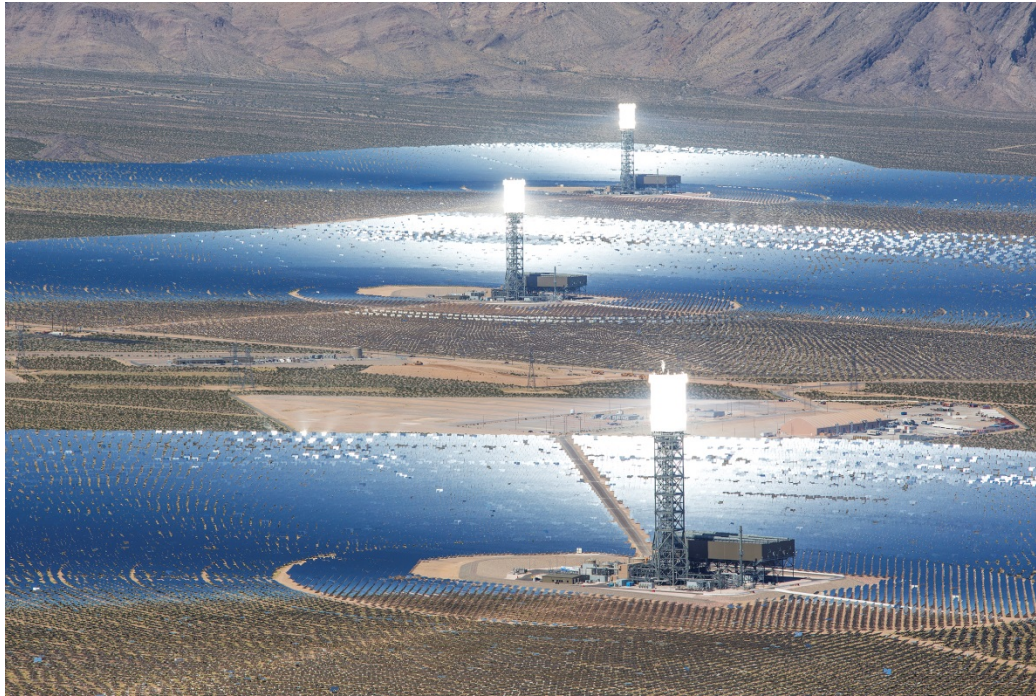
Figure 4. The Ivanpah Solar Electric Generating System (source: BrightSource Energy)
