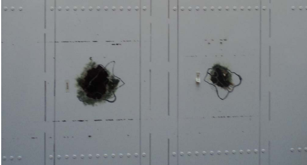
Fig. 2. Structural damage in the outer skin in the Airbus A400 M airplane after the lightning strike
