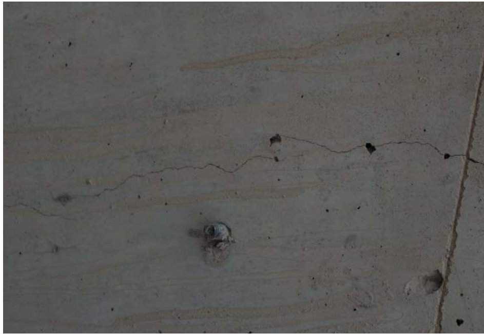
FIGURE 1: Cracks on the concrete surface.
