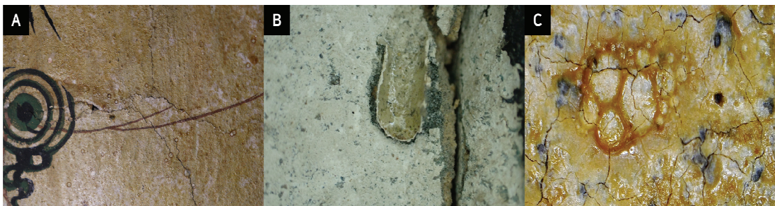
Figure 14. Damage caused by presumed to be the fixative (A: Crack, B: Delamination, C: Gloss).
