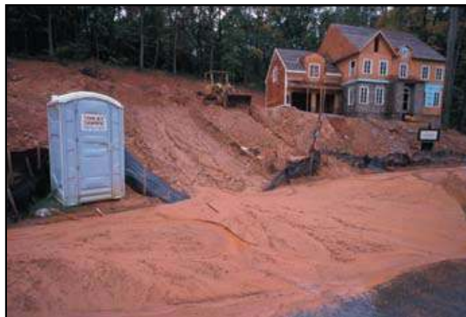
Sedimentation, a pervasive form of aquatic habitat degradation throughout much of North America, here results from poorly regulated construction in the Nancy Creek system, a Chattahoochee River tributary in metropolitan Atlanta (1997).
