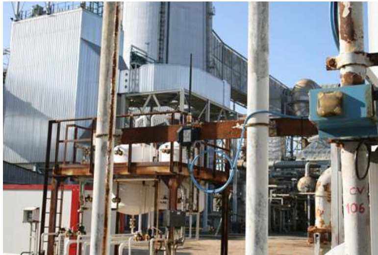
Fig. 1: Sensor Node in the Petrogal oil refinery in Sines, Portugal.
