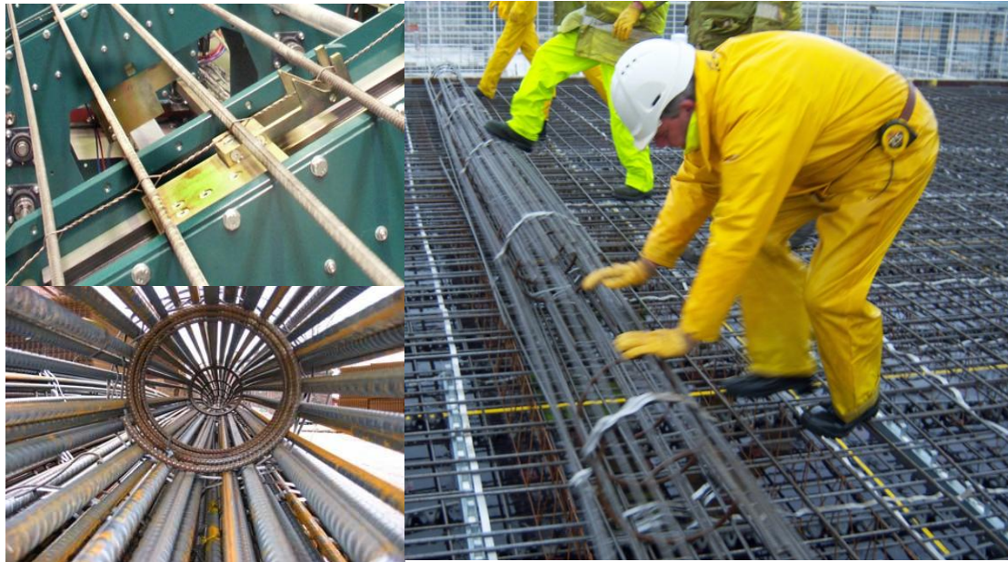
Figure 6 - Fabrication of the SpinMaster reinforcement roll in the factory and the installation on-site. (Celsa Steel Services, 2013)
