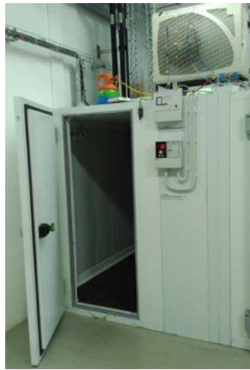
Figure 2. Walk-in freezer in the laboratory of AKO ELECTROMECAÁNICA S.A.L.
