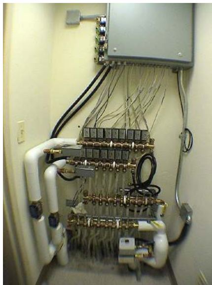
Figure 15: Hydronic Heating Manifold and Control Valves
