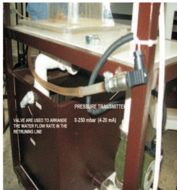
Fig. 4. Photo of pressure transmitter and valve
