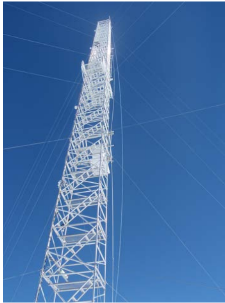
FIGURE 4.3 – The 45 m tower at Dome C. Photo C. Brun.
