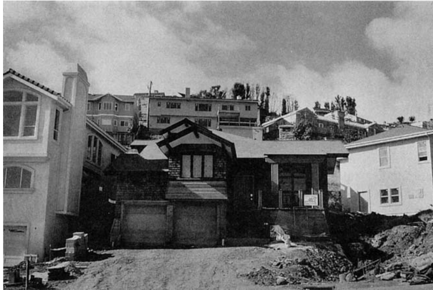
Photo 10.3 The rebuilding process has produced eclectic variety in house styles, built in extreme proximity to one another
