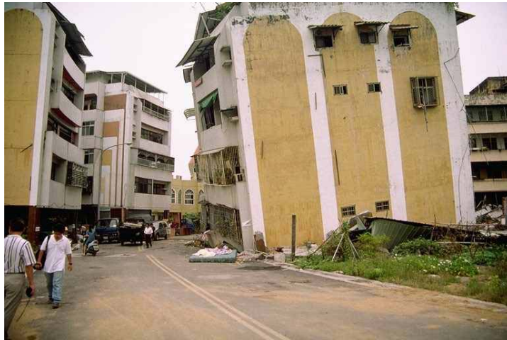
Figure 3. Photo P-2 showed the collapsed 6-story reinforced concrete building in Wufeng Site A (by R. Seed, 1999)
