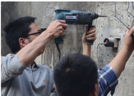
FIGURE 3: Simulation of partial damage in the wind-break wall.
