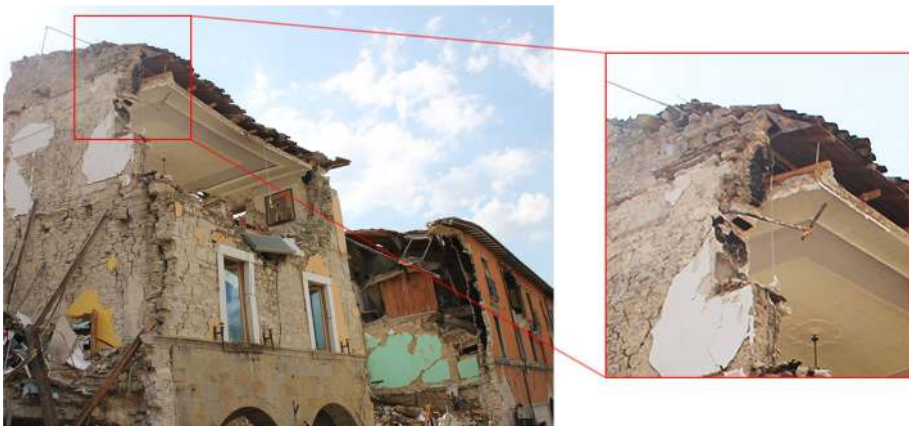
Fig. 14 Partial facade collapse (mechanism M3) of a building which had tie rods: general view (left) and detail (right)
