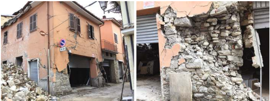
Fig. 23 Residential masonry building: D4 damage level, shear failure of external walls mechanism (M1), poor masonry vulnerability factor (ev4)
