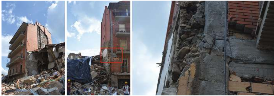
Fig. 27 Residential RC building (damage level D3): global damage (left), damage of beam-column node (center), particular of the node (right). Damage mechanism MC, vulnerability factor e_vD
