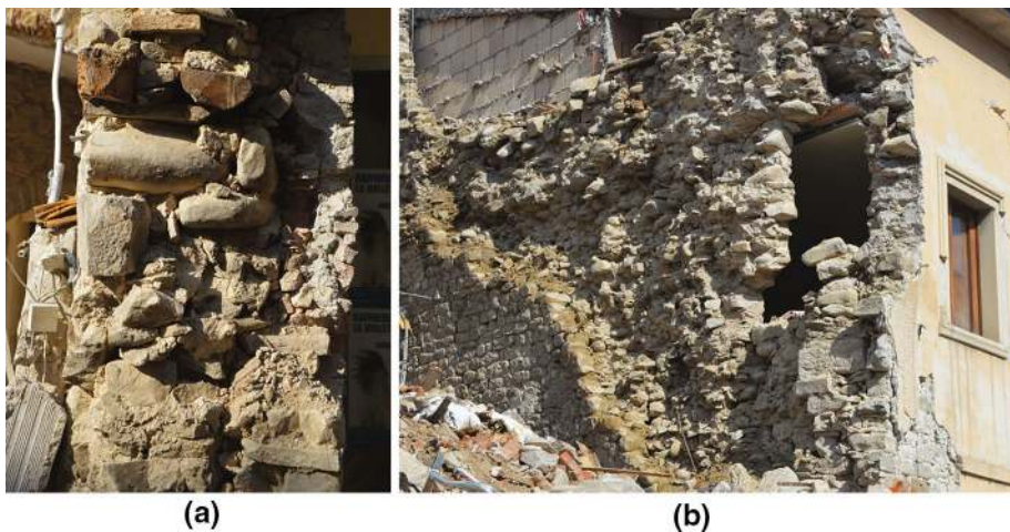
Fig. 18 Example of ev4 vulnerability factor (poor quality masonry): a absence of bondstones in the wall-section; b cobblestones with poor quality mortar
