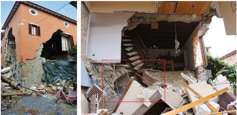
Fig. 24 Residential masonry building: D5 damage level
