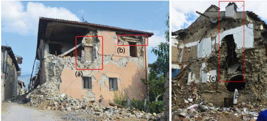
Fig. 19 Example of ev12 vulnerability factor (local discontinuities): closure of previous wall openings (a), presence of weak wooden elements (b), presence of chimney in the wall (c)
