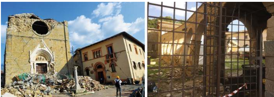
Fig. 26 Church of S. Francesco: damage level D4, collapse of tympanum (M6) and in-plane cracking of façade (left); collapse of columnnade (right), ev1 vulnerability factor
