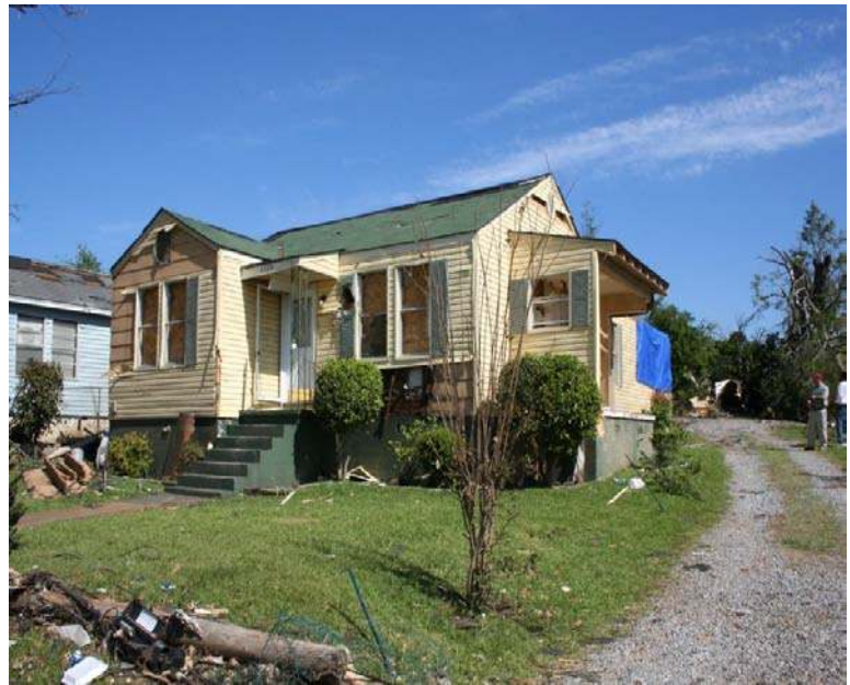
Figure 4.12 Loss of a wall
