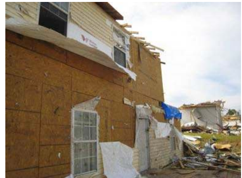
Figure 5.3 Loss of siding material
