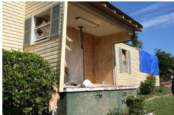
Figure 4.11: Single family dwelling with moderate EF/damage
