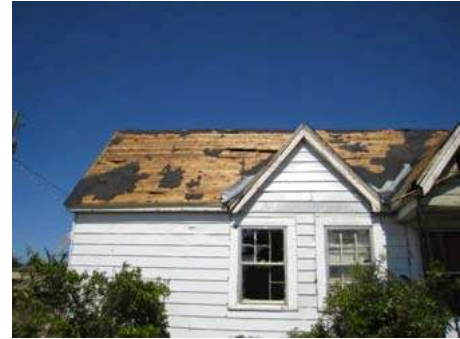
Figure 5.2: Loss of roof covering
