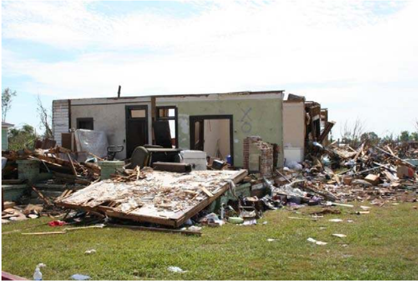
Figure 4.5 Interior walls collapsed
