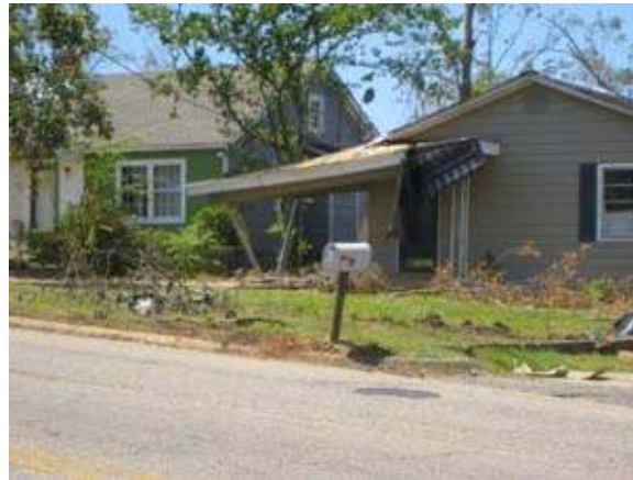
Figure 5.8 Porch or carport damage
