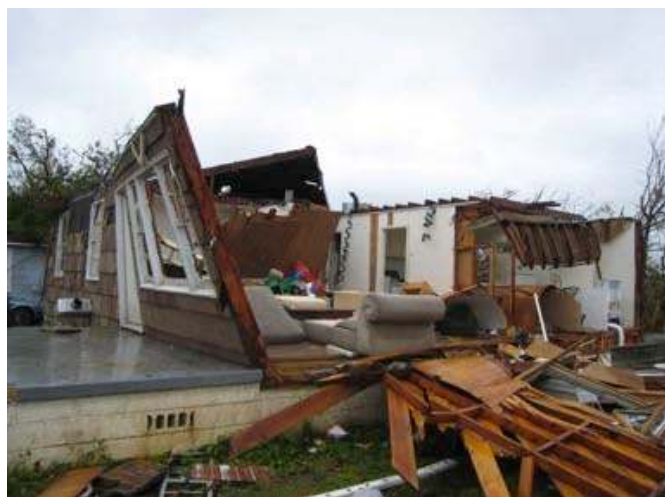
Figure 5.11 Exterior walls collapse
