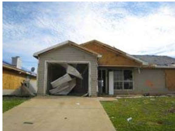
Figure 5.7 Garage wall blown-in
