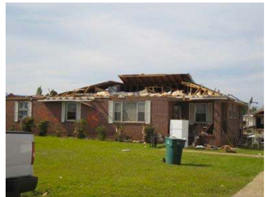
Figure 5.5 Significant roof damage
