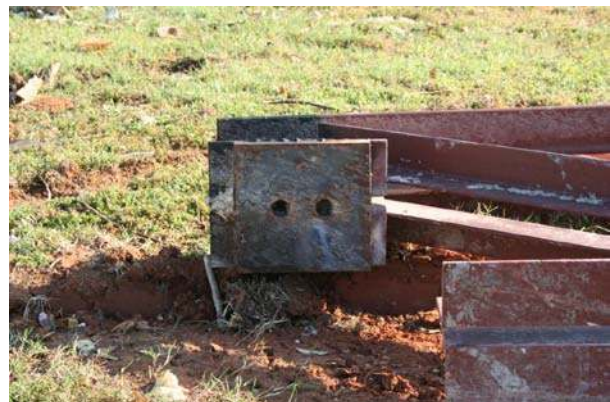
Figure 4.16: Roof truss that was lifted off during tornado; diagonal member buckled (not shown here).
