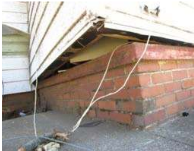
Figure 5.9 House shifting off the foundation
