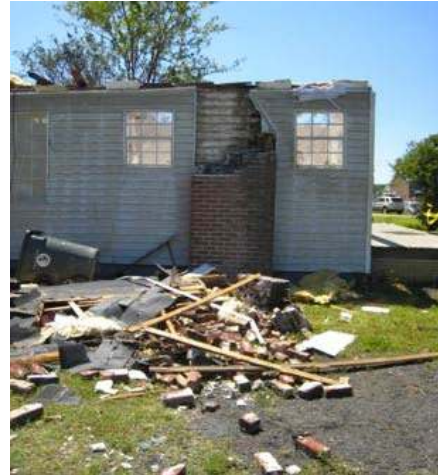
Figure 5.6 Collapse of chimney
