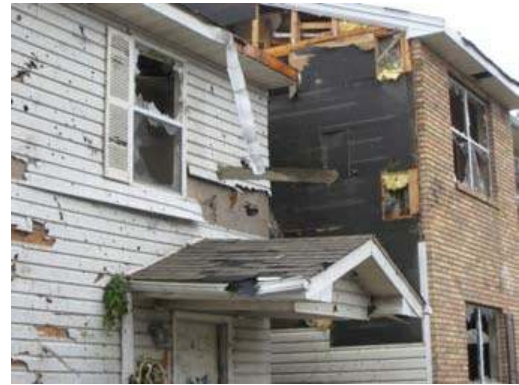
Figure 5.4 Broken windows and doors
