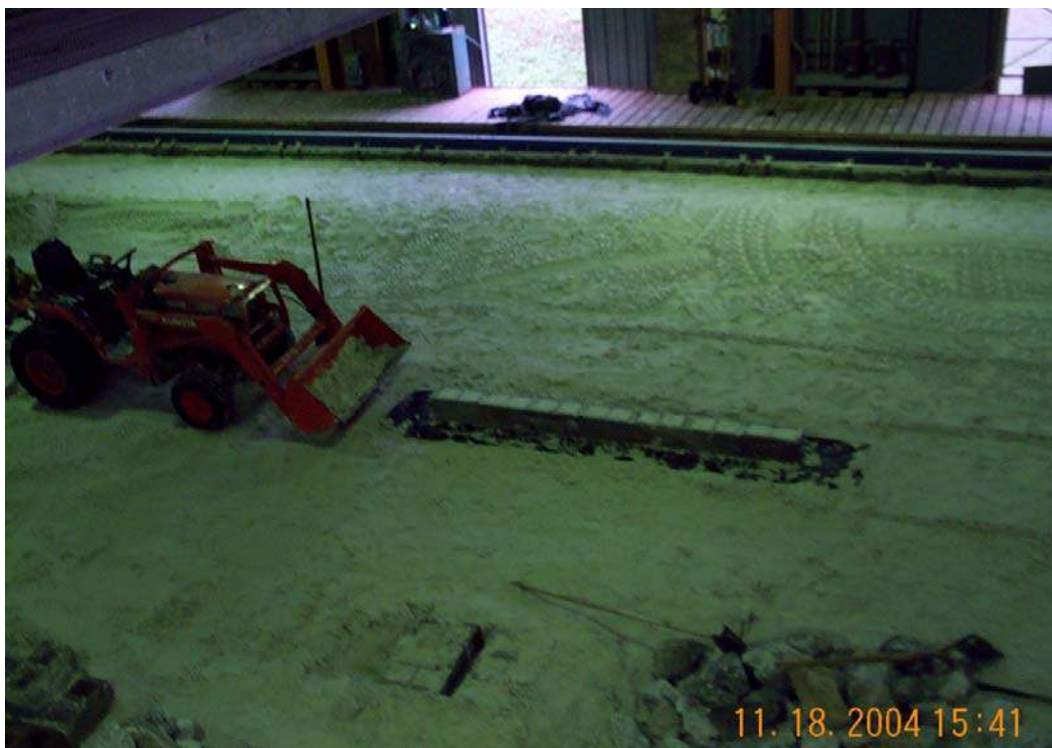
Figure 143. Nearshore breakwater with filter cloth covering foundation layer and second row of sand-filled blocks.
