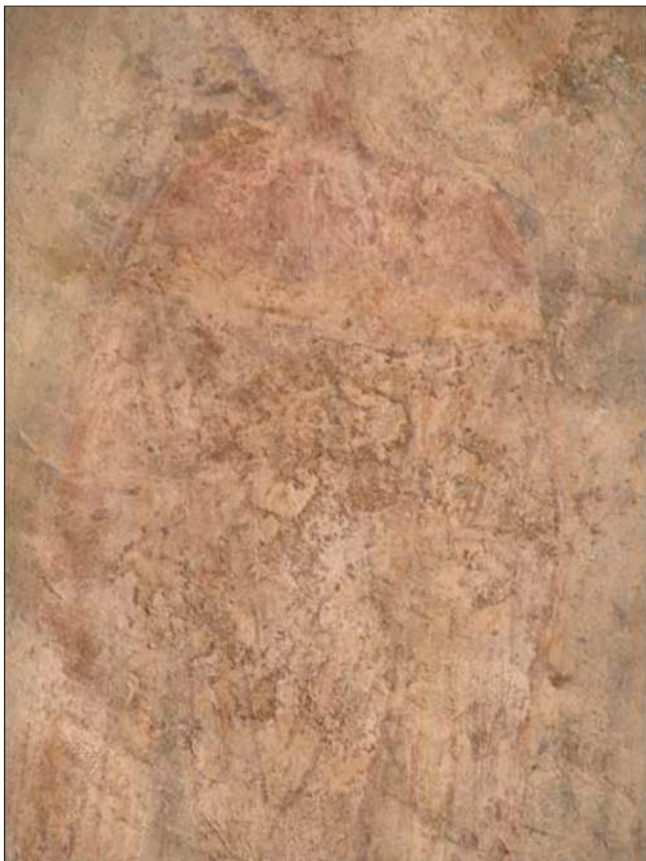
Figure 6. Hands of the Virgin Mary. Detail of parts of the mural which have fallen out, salt efflorescence and mold (photo from author's archive).
