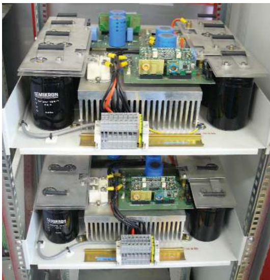
Fig. 8. 5 kVA single-phase two-cell SDC-CHB prototype.
