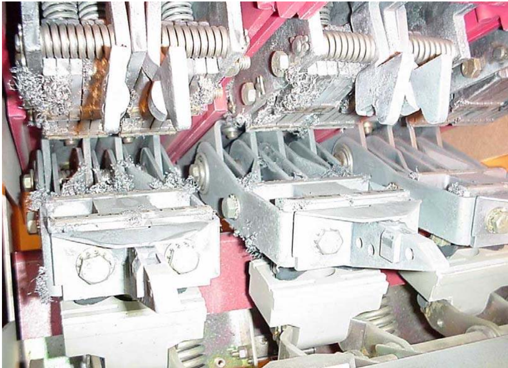
Fig.1. Silver whiskers inside circuit breaker in May 2000 (before cleaning)
