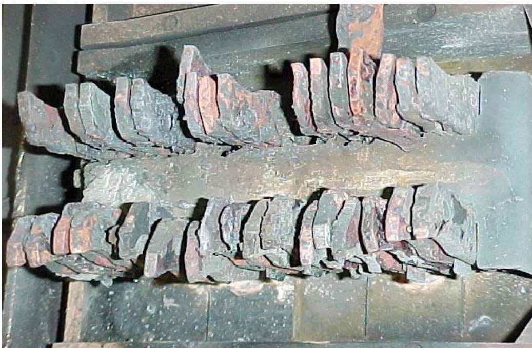
Fig.2. Finger Cluster after failure in July 2000
