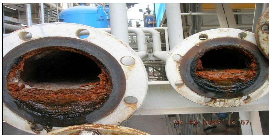
Figure 8. Fouling effect in the pipe line of gas sweetening plant (ARIANA, 2010; Internet, 2010a, 2009).
