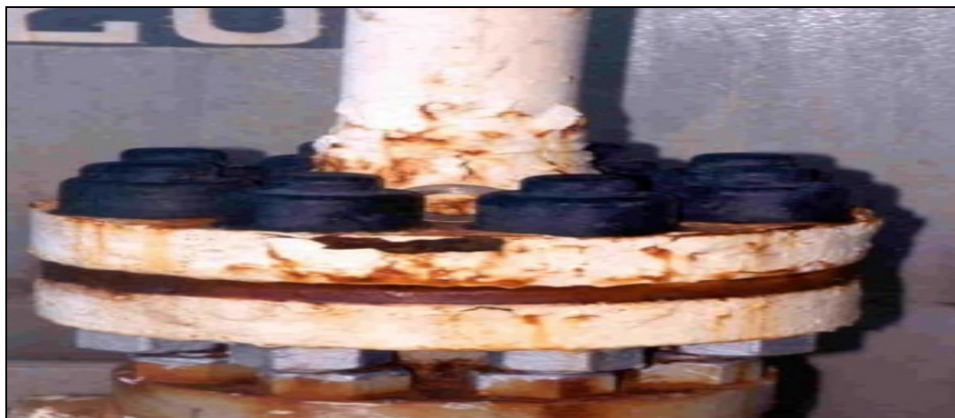
Figure 6. Crevice corrosion in the junction of pipelines (CTL, 2010).
