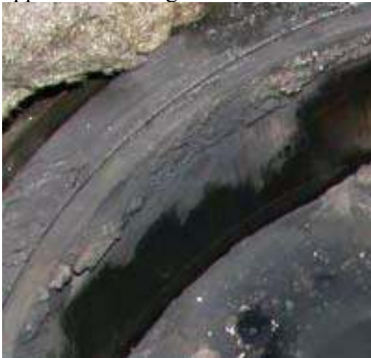
Figure 3-45 Severe flame ring deposits.
