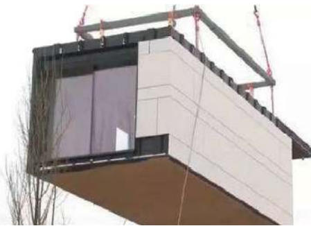
FIGURE 2: Hoisting and installation of a modular prefabricated building prototype (source: authors' own data).
