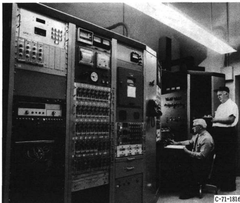
Figure 7. - Test control room.
