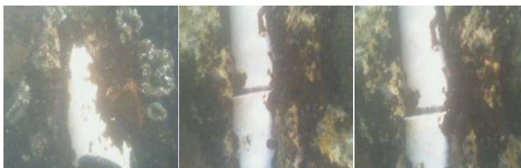
Figure 24. Images of incrustations on underwater PVC pipes.
