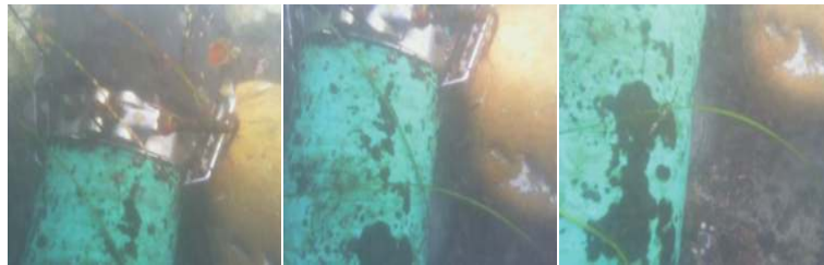
Figure 21. Underwater images of PVC pipe fasteners.
