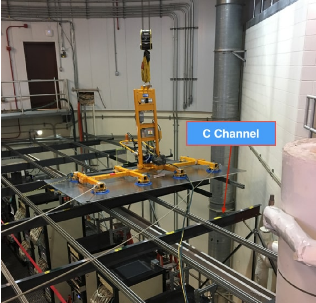
Figure 17: MicroBooNE top plane support structure and C Channel. The roof crane and rigging system is placing one module in position.
