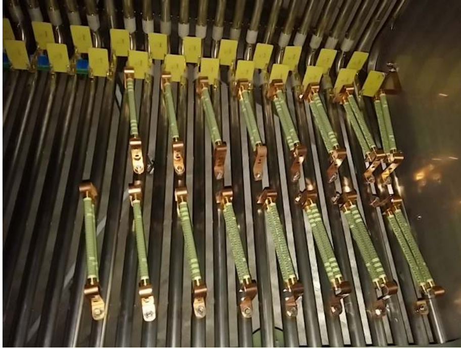
Figure 16. The Metallux HVR 969.23 resistors mounted on the 16 field cage loops closest to the cathode.
