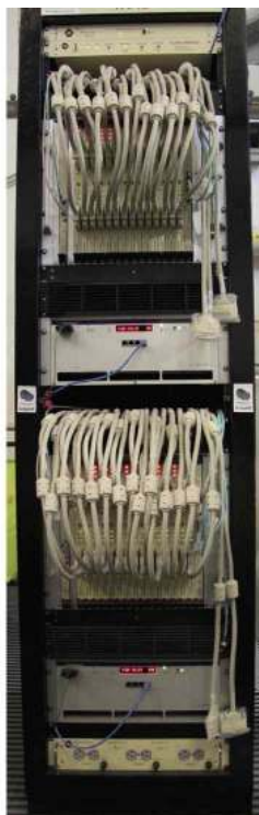
Figure 54. Rack containing two of the nine MicroBooNE TPC readout crates.
