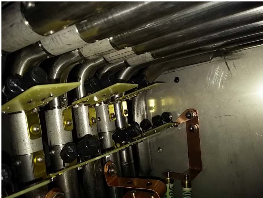
Figure 17. Surge-protecting varistors (small black disks in the photograph) are installed in parallel with the voltage divider resistors for the first 32 field cage loops. Here, they are shown mounted on small boards in sets of 3, and attached to the field cage by means of 6-32 hex-head button-screws.
