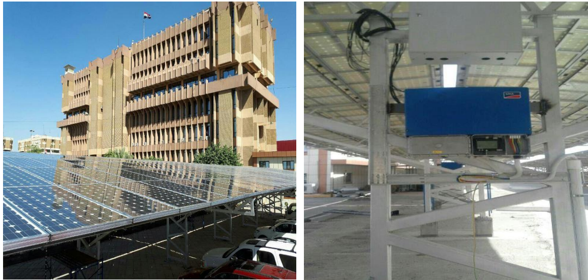
Figure 4. This figure shows the real PV system grid tied that has been installed at Baghdad Site, (a) Solar Array (Sharp 175Wp); (b) Solar Inverter (SMA 25kW).
