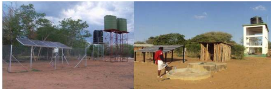
Figure 5. Water pumping stations driven by PV systems for human consumption in Mozambique.
