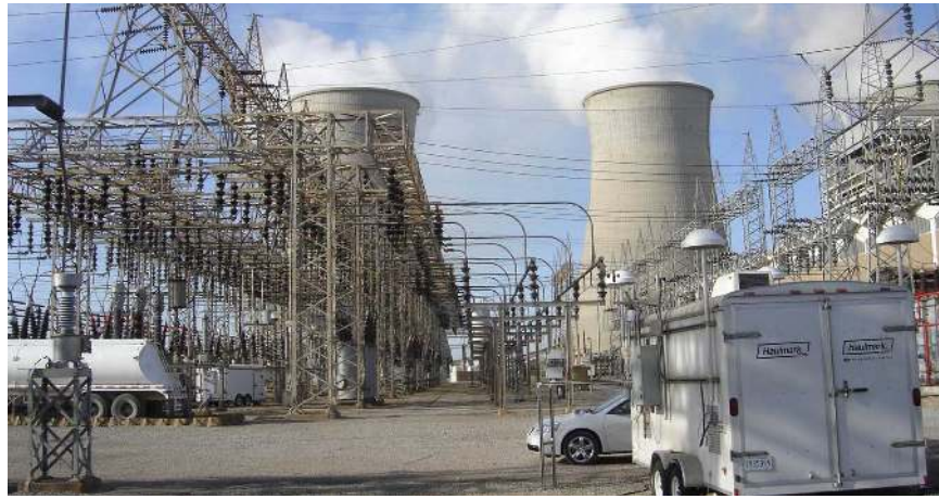
Fig. 1. View of the Paradise substation, showing the trailer that houses the current base station located at one end of the substation.
