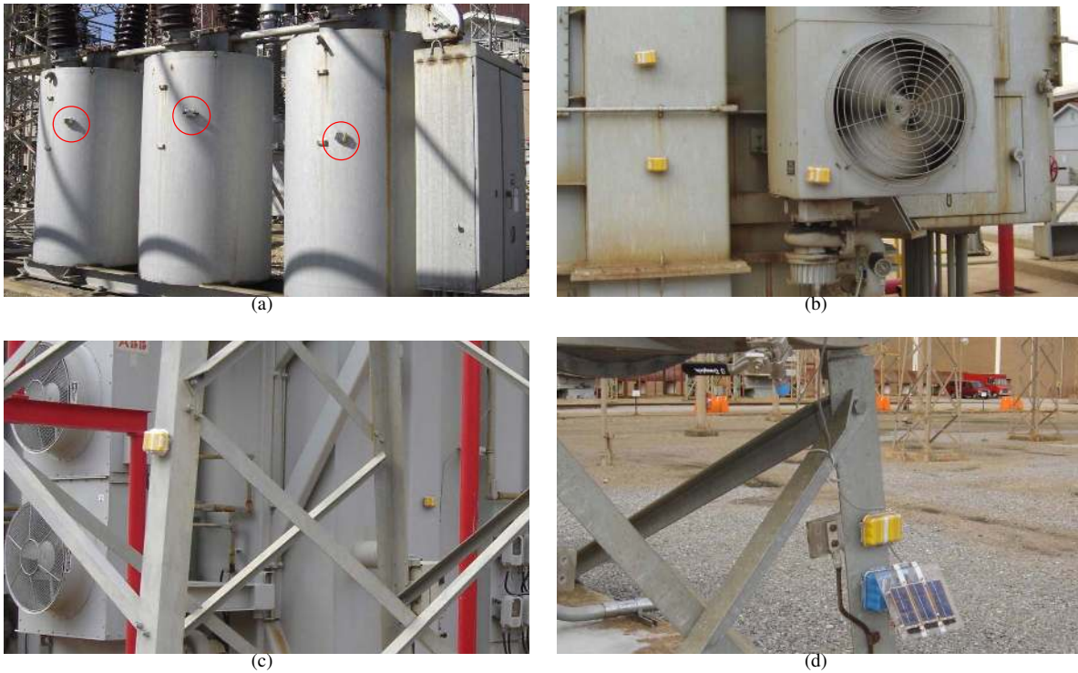
Fig. 2. Illustrations of wireless sensor nodes deployed in the Paradise substation: (a) surface temperature sensors for oil-filled circuit breakers, (b) temperature, vibration, and sound intensity sensing from oil-cooled transformers, (c) ambient temperature sensors, and (d) a solar-powered SF_6 gas density sensor node.
