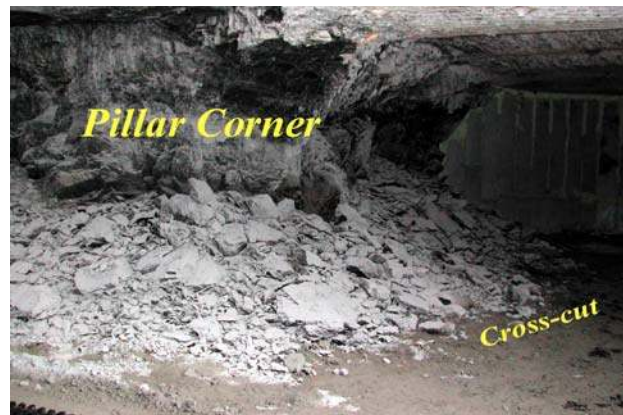
Figure 5-4 A photo for a failed pillar corner
