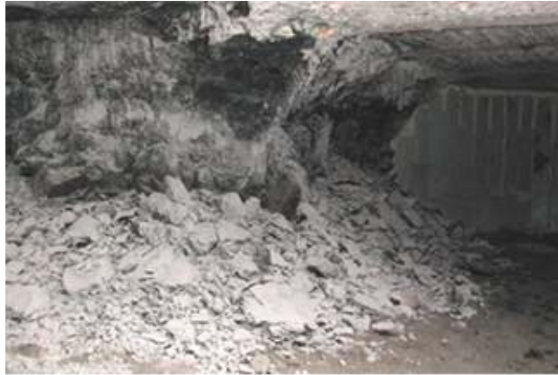
Figure 6-12 Rib's sloughing at 2200 ft deep
