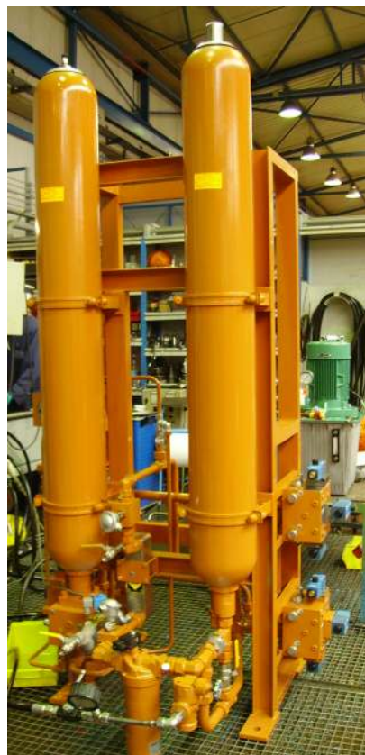
Figure 7. HP and LP accumulators.
