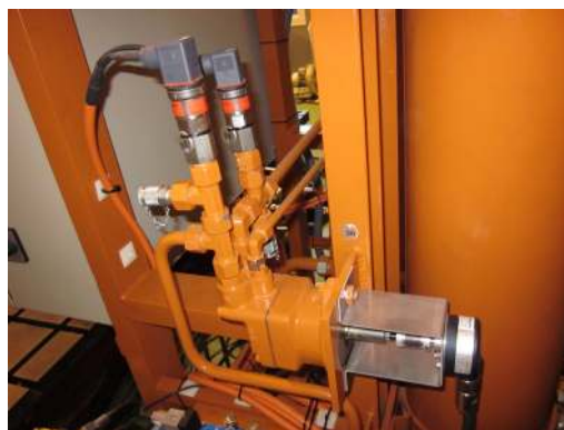
Figure 9. Hydraulic motor, input and output pressure transducers and the encoder coupled to the shaft.
