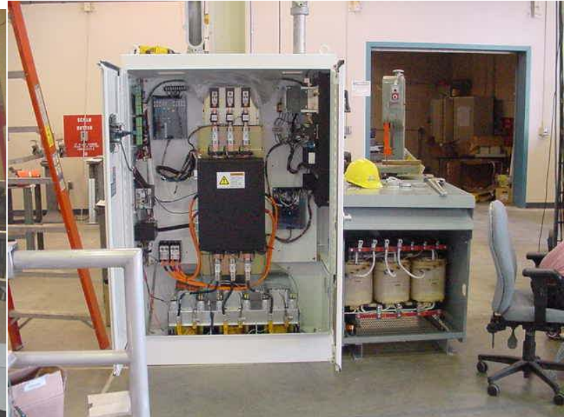
100 kW system test at Ballard Power
