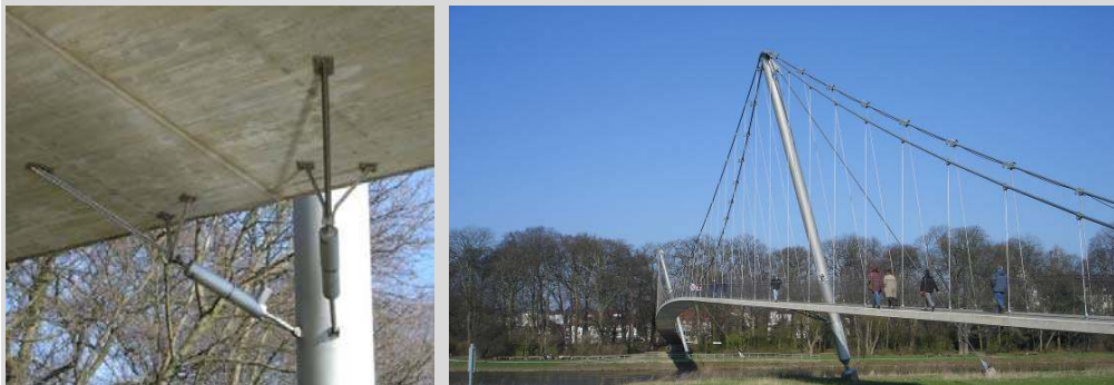
Figure 6-2: Viscous dampers installed at Minden footbridge (Germany)
