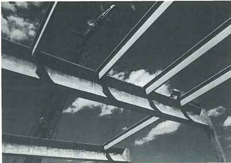
Fig. 18. Purlins framing into curved prestressed beams which used Cazaly hanger type connections. This framing system was used for many warehouses.
