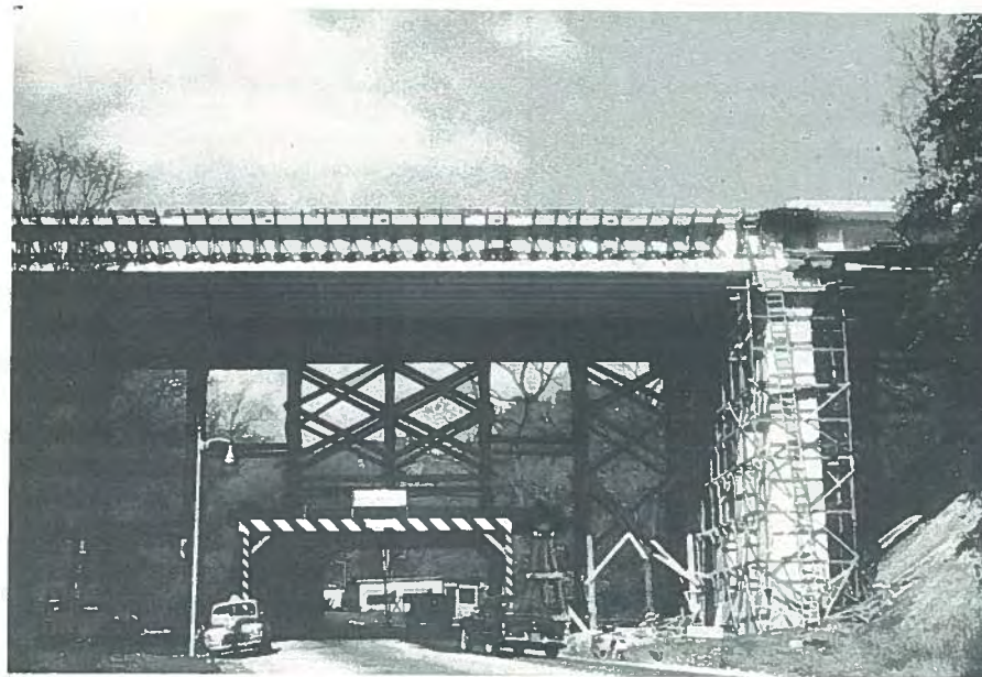
Fig. 1. The Walnut Lane Bridge under construction in 1950. Photograph shows brackets in place for formwork for sidewalk at south fascia girder.
