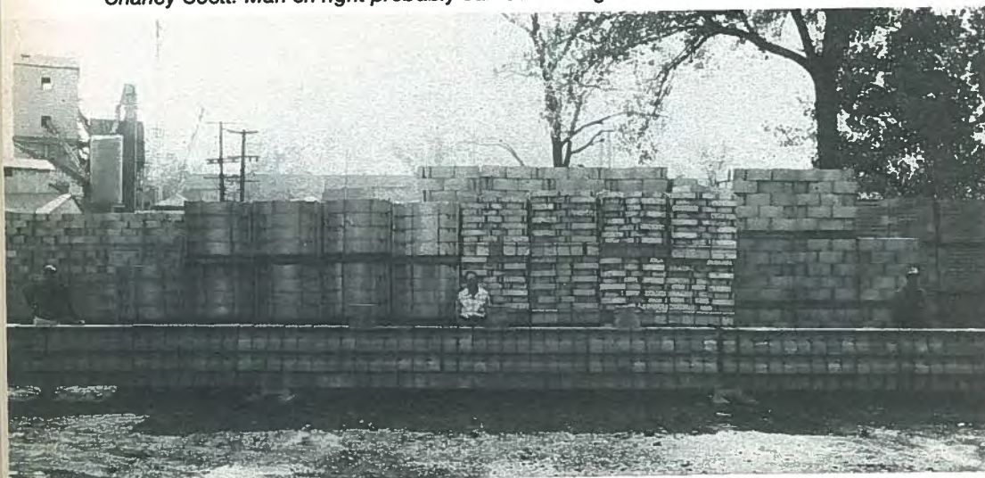
Fig. 17. Continuity test at Breeko Plant. On the left is Lloyd Markham, at center Charley Scott. Man on right probably carried loading blocks. Taken in August 1952.
