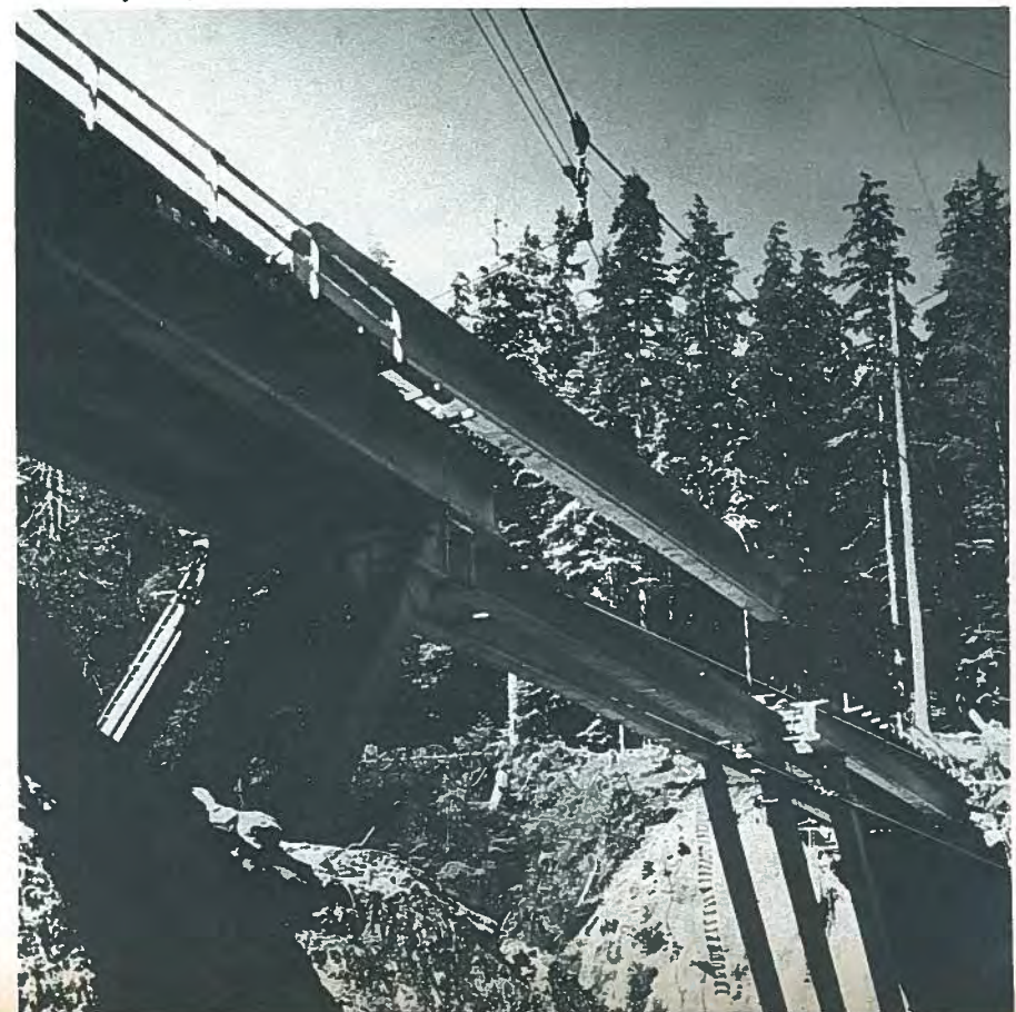
Fig. 80. The deck bulb-T being used advantageously at a remote mountainous site. Over the years, this section has found extensive use in the rugged northwest.
