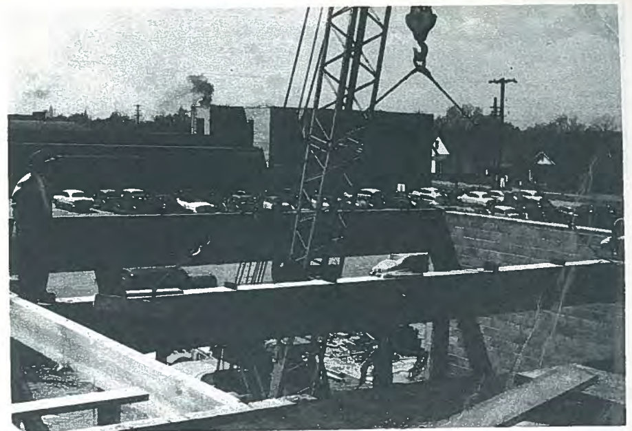
Fig. 14. The largest prestressed beam in Colorado made by Prestressed Concrete of Colorado was for the Plat Packing Plant in 1952.
