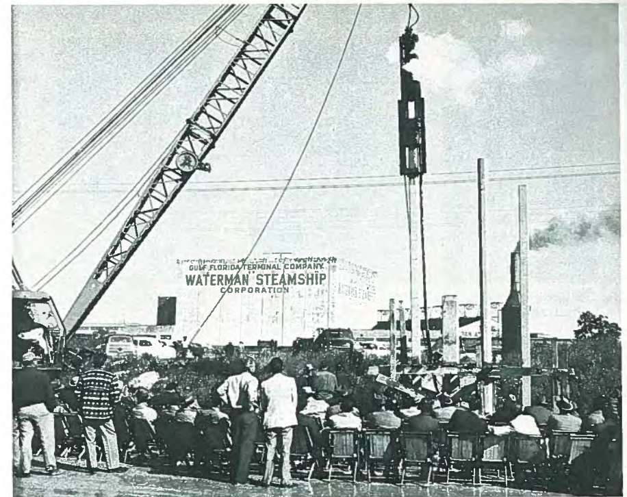
Fig. 32. Pile driving demonstration test of series of piles at Cone Brothers Construction Co., Tampa, Florida. Courtesy: Paul Zia.
