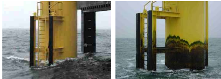
Figure 3.8 Marine growth at OWEZ met-mast, one year after installation
