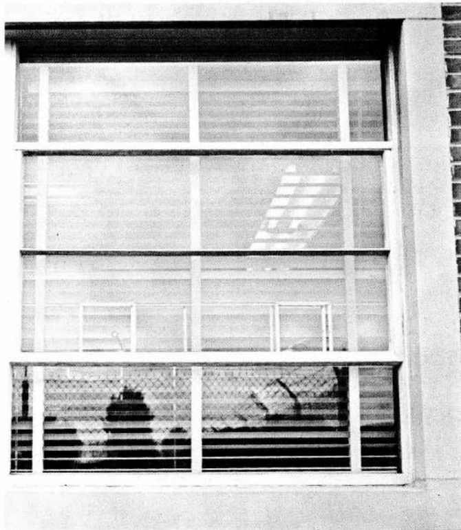
Figure 2. Typical window at USACRREL.
