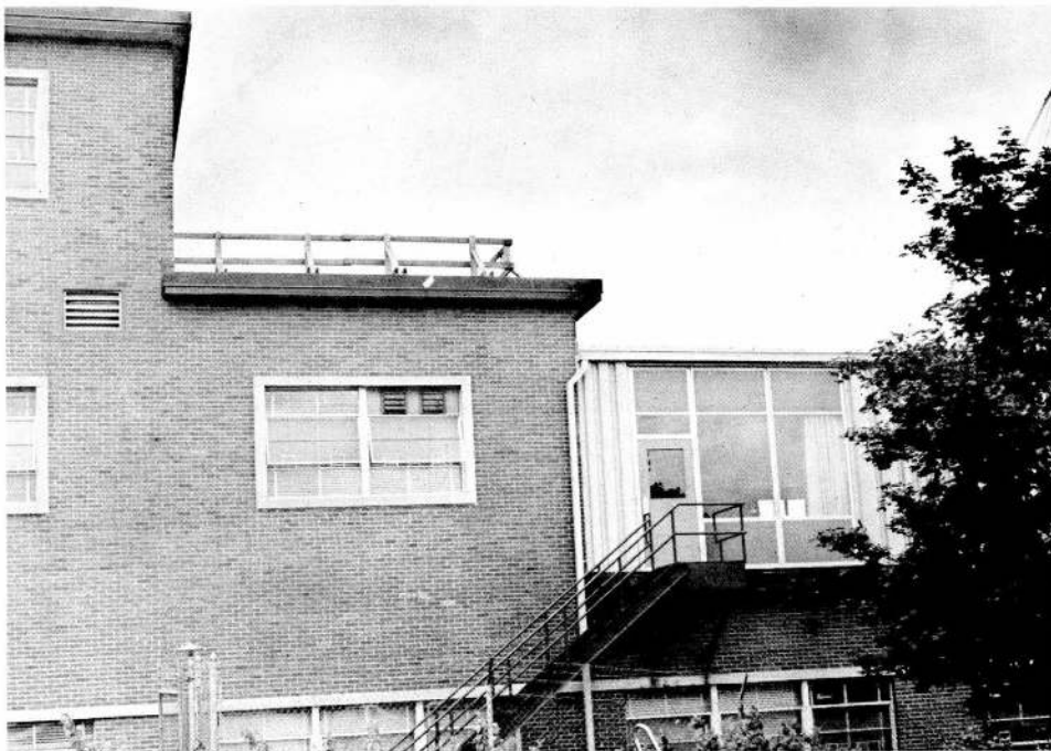
Figure 8. West side of north-facing wall. Lower arrows point to heat escaping by conduction through wall of the cafeteria kitchen. Upper arrows point to heat escaping by conduction through wall of second floor office. White arrows point to location of heat leak (see Fig. 7).
