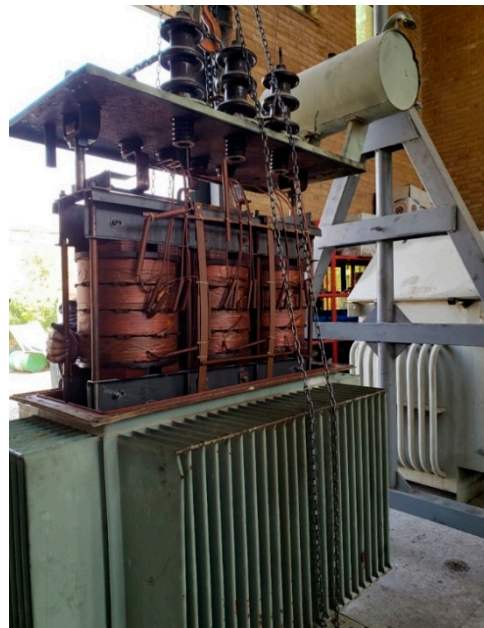
Figure 2. The three-phase distribution transformer under testing.
