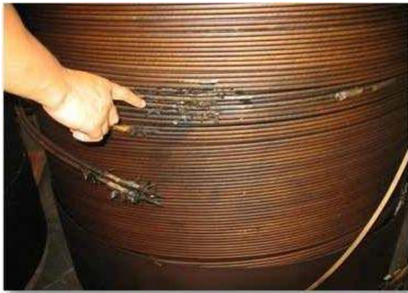
Figure 10 : Damaged LV (phase-C) coil
