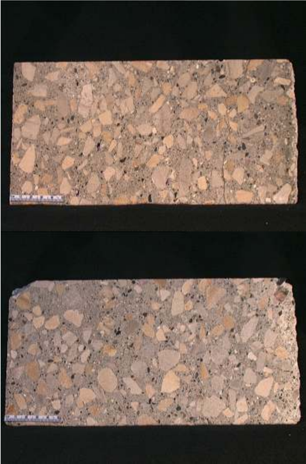
Figure 38. Cores 11, joint (top) and 12, mid-panel (bottom) cross section with horizontal crack in lower-most third. Some segregation is visible in both cores.
