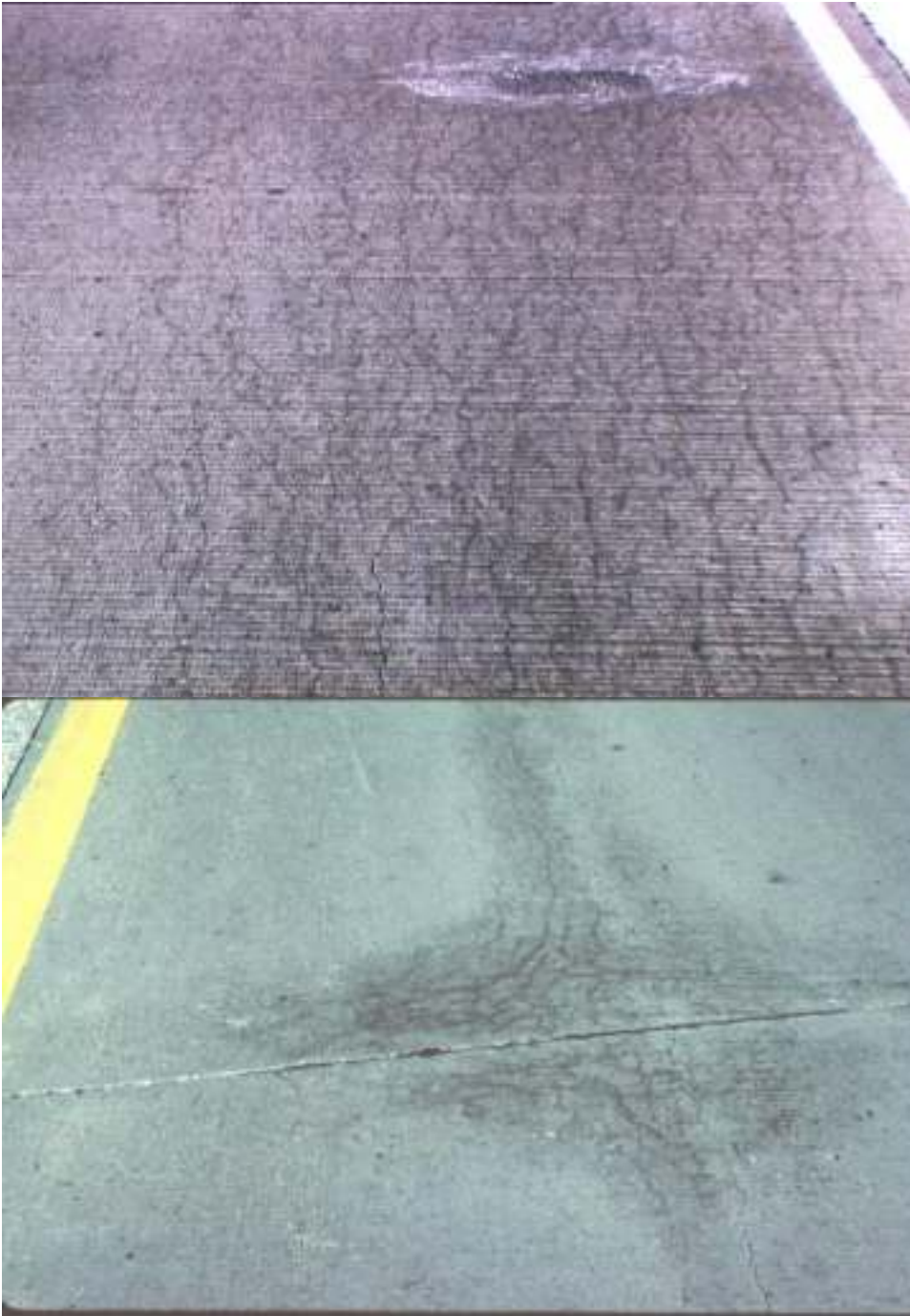
Figure 2. Map cracking oriented in the longitudinal direction of the pavement, interconnected by slightly finer cracks perpendicular to pavement direction becomes more prominent with progression of deterioration (top). Advanced degradation shows cracking paralleling the transverse joint and road edge, and along cracks within vibrator trails. The degradation would be characterized initially as “low” severity according to the SHRP Distress Identification Manual [17] and “moderate” as the deterioration progresses.
