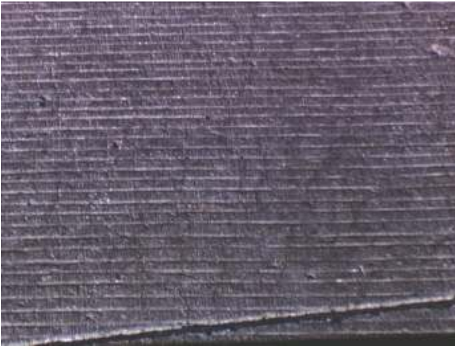
Figure 1. Onset of pavement deterioration is visible as a slight darkening of the concrete in the transverse joint region (top, I-80) and in pavements with advanced deterioration, a tightly-closed pattern cracking (bottom, US 20). Some of these pavements also have vibrator trails.
