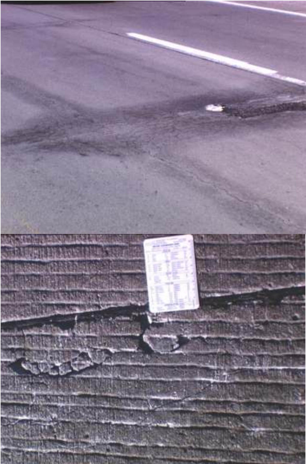
Figure 3. Pavements exhibiting severe deterioration show significant pattern cracking (here accentuated by moisture along the crack), cracking along joints, spalling along joint edges and white efflorescence. Open joints and lack of displacement along pavement slabs provides evidence against permanent expansive processes such as alkali-aggregate reaction and sulfate attack.
