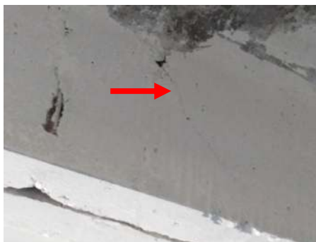
Fig. 2. Crack in the edge of the slab. Opening width up to 0.4 mm.
