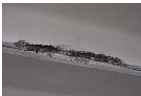
Fig. 3. Bare reinforcement and its surface corrosion with the destruction of the protective layer of concrete.
