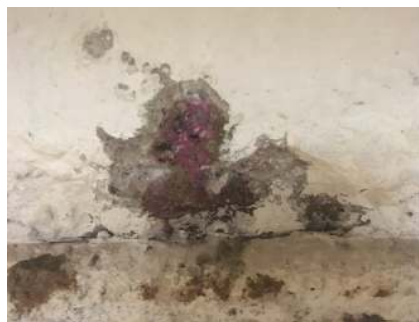
Fig. 6. The depth of carbonization according to the visual data of the phenolphthalein sample exceeds the value of the concrete protective layer by 10 mm, according to the autopsy data No. 7.
