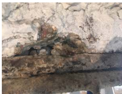
Fig. 5. The absence of visible signs of concrete carbonation according to the results of phenolphthalein samples in the areas behind the working reinforcement according to autopsy No. 2. No concrete protective layer is present.
