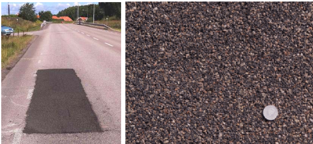
Figure 3 – The Swedish pilot test track in Linköping; on-site construction (pictures: U. Sandberg, VTI)
