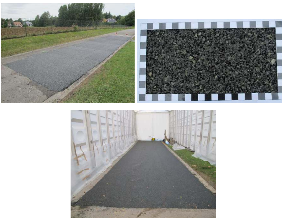
Figure 5 – The Belgian pilot test track in Sterrebeek; on site construction: Sterrebeek I (two top pictures) and Sterrebeek II, which had to be constructed under a tent due to the cold and wet season (lower picture) (size of black/white squares is 10 mm) (pictures: A. Bergiers, BRRC)
