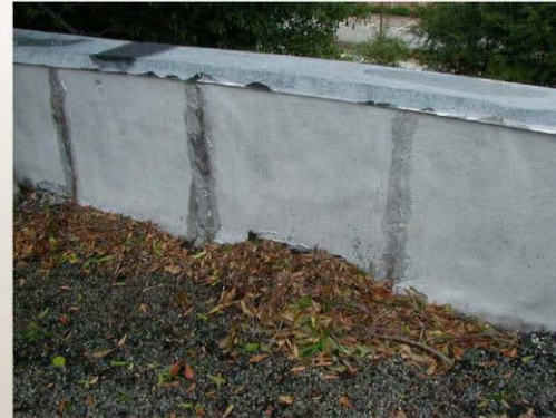
Rain/drainage: blocked scupper
