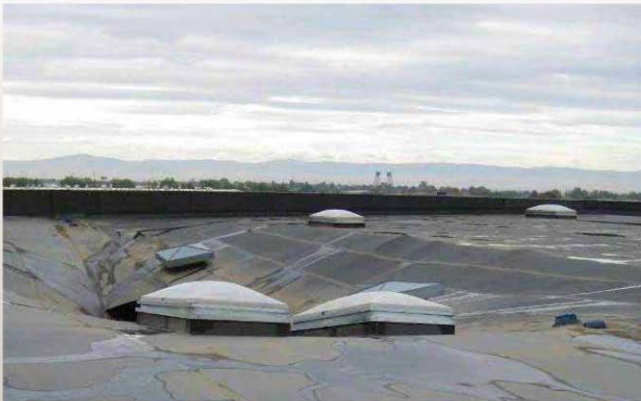
Partially blocked drains, slope
