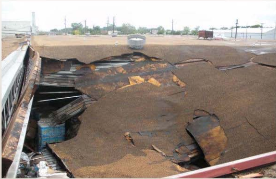
Rain/drainage: soaked cover boards and ponding
