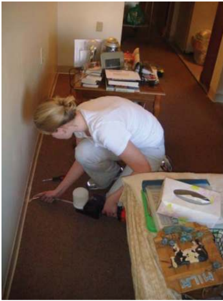
Fig. 4. A diatomaceous earth barrier was applied underneath the vinyl baseboard around the perimeter of each apartment unit using a power duster. Pictured is the Exacticide Power Duster.
