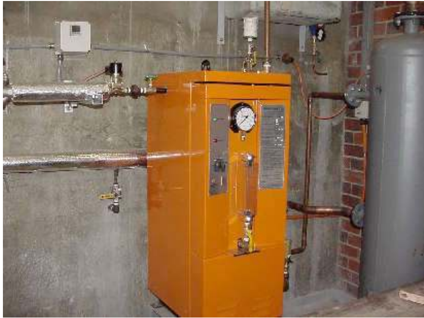
Figure 3.13: Steam Boiler and Controls
