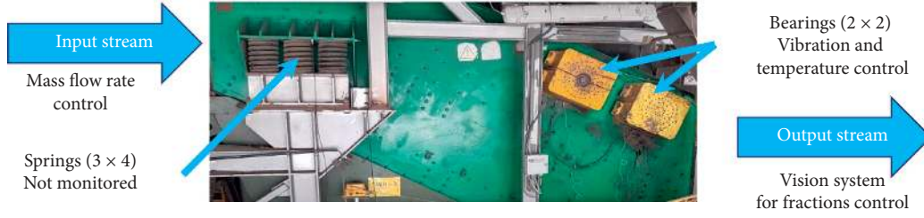
FIGURE 3: Components of the monitoring system on the vibrating screen (nondriven side) with two exciters.
