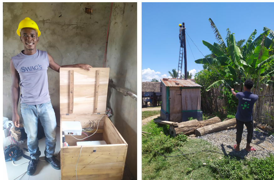
Figure 28. Installation of the interconnection modules in Ambohimena and cable connection at the top of a pole.
