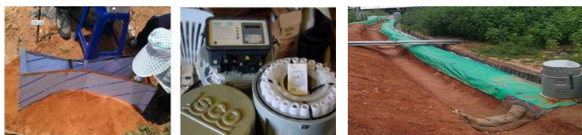
Figure 4. Installation of parshall flume and automatic sampler (left) and hybrid BMP within a ditch (right).
