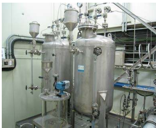
Figure 4. Water chemistry balancing system.
