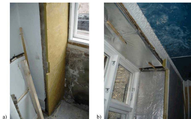
Fig. 7. Insulation applied in the window reveals where (a) is Aerowolle and (b) is Vacupor NT.
