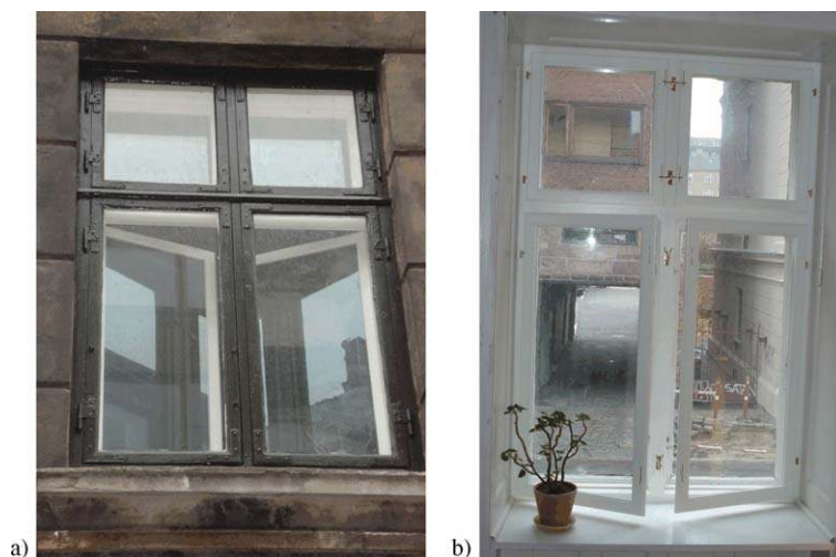
Fig. 4. Energy retrofitted 4-light Window 2 with a secondary frame seen from (a) exterior of building and (b) interior.
